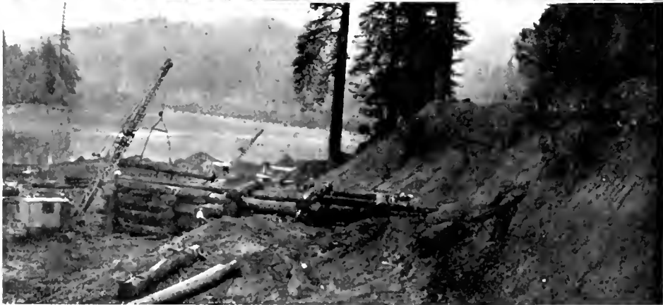
Pictures of deflector construction with 27-inch redwood logs from the foundation excavation to the completed structure filled with screened gravel of two-inch minimum size
